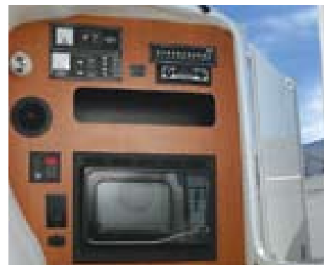
Forward cabin bulkhead houses the stereo controls, shore power panel, circuit breakers, AC controls, 120 V receptacle and microwave.
