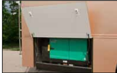
Onan Quiet Diesel Generator Upgrade
