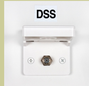
Auxiliary Cable/Satellite input & exterior coax output.
