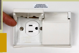
Exterior GFCI 110V Outlets.
