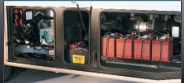
There's easy access to the 2,000-watt power inverter and all of Bounder Diesel's batteries.
