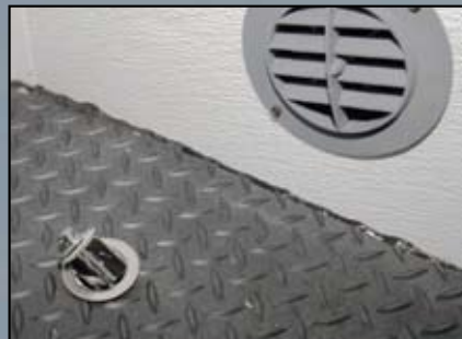
Floor drain and ducted heat in garage
