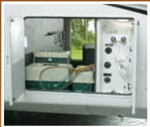
Enclosed utility management compartment
