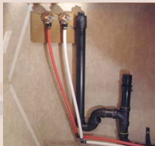
All GRAND JUNCTIONS are prepped for washer/dryer.
