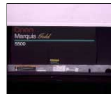
5.5 kW Onan generator
