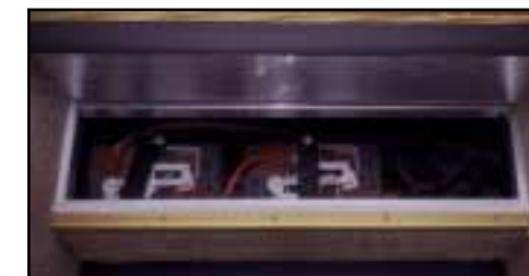
Battery access in step
