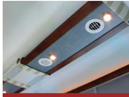
Set at the peak of the crowned roof, a stylish soffit provides ducted A/C and central lighting
