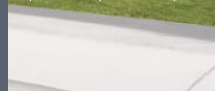
One-year-old Winnebago Industries' fiberglass roof
